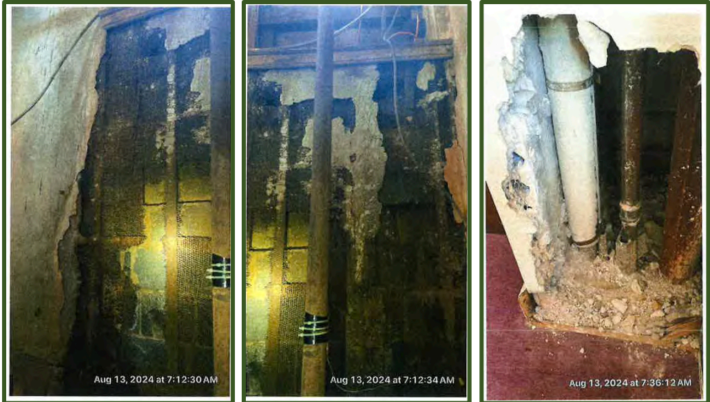
Figures 49-51: Images of significantly damaged materials within Taylor Hall, both finishing and structural, resulting from water damage 12
