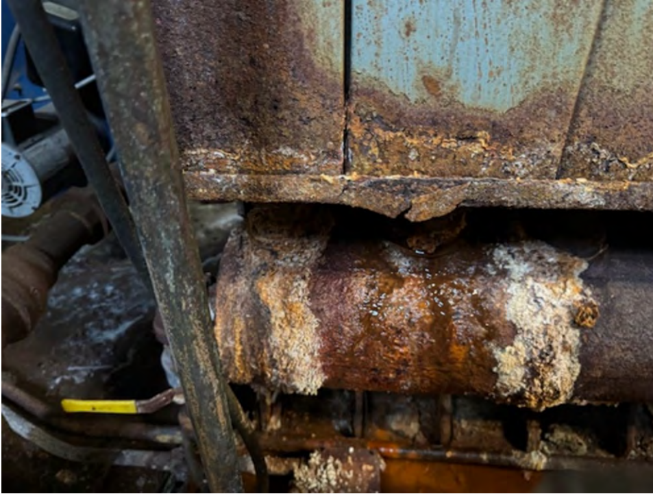
Boiler #2 Mud Drum Leaks - Multiple Failures
