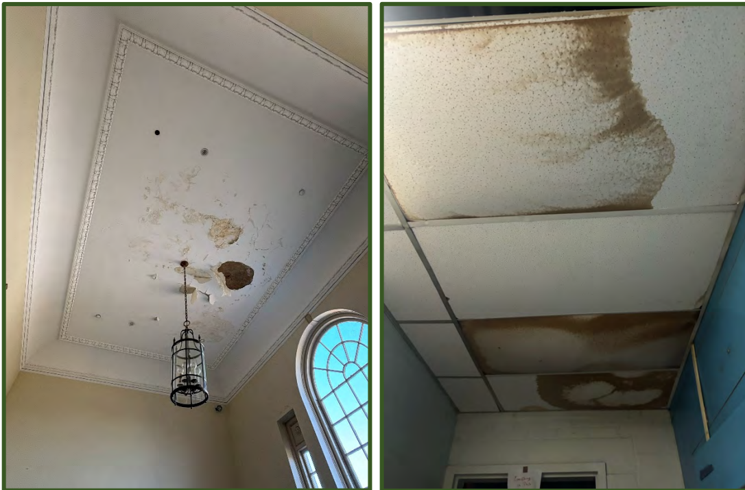
Figure 43 (left): Damaged plaster on the ceiling of Bristol Hall.
