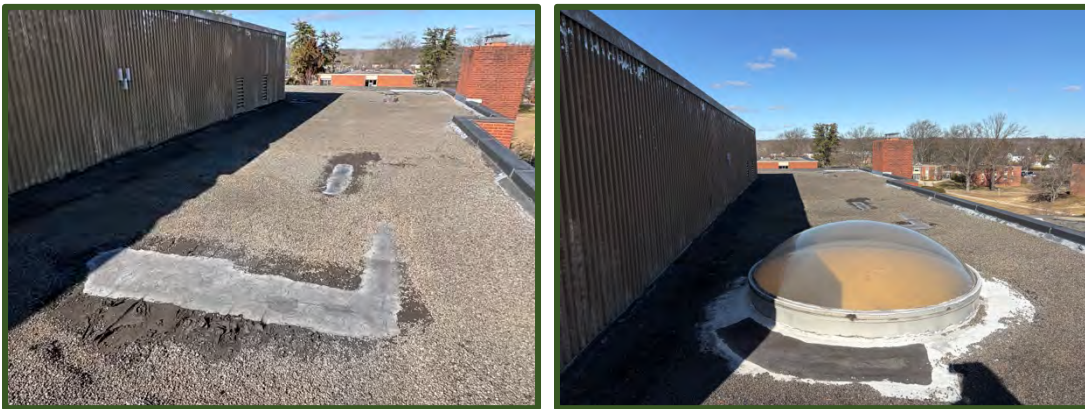
Figures 59-60: Roof of Student Center, depicted patches which signify poor roof conditions
