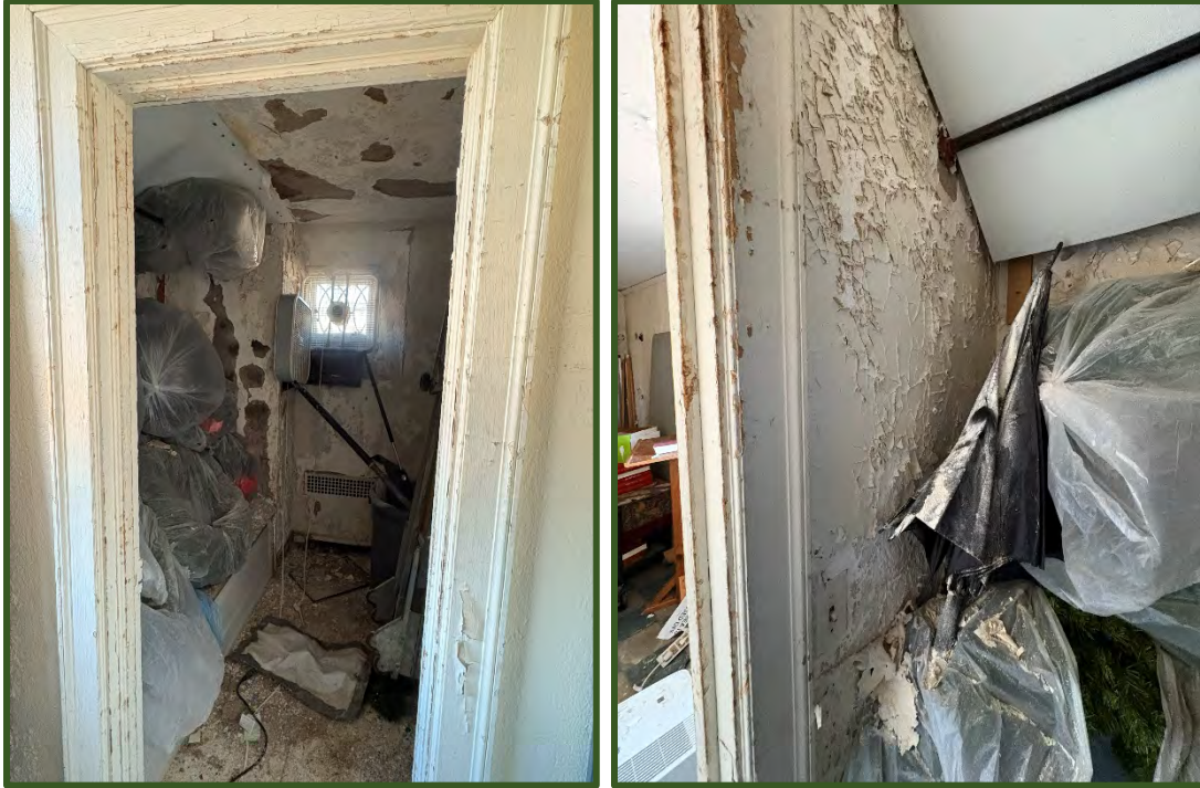
Figure 41-42: Steam damage depicted in Bristol Hall.
