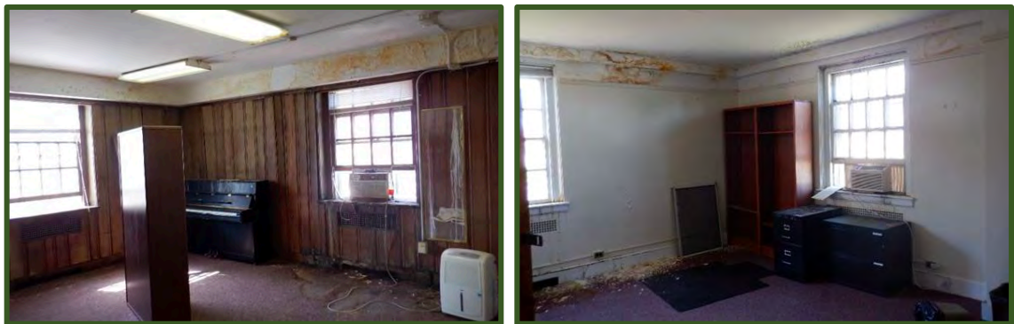
Figures 52-53: Steam damaged room in Taylor Hall 13
