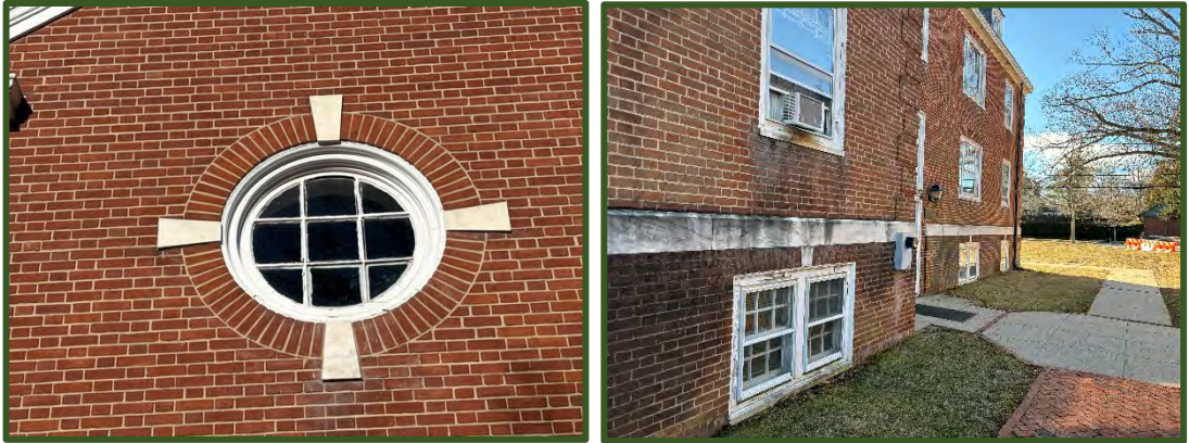
Figure 62 (left): Exterior rotted window at Bristol Hall. Figure 63 (right): Exterior rotted windows in Erdman Hall.
