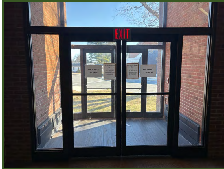
Figure 27: Exit/Entrance stairs which depict accessible exit with no sidewalk. Signs read "EMERGENCY EXIT ONLY!"
