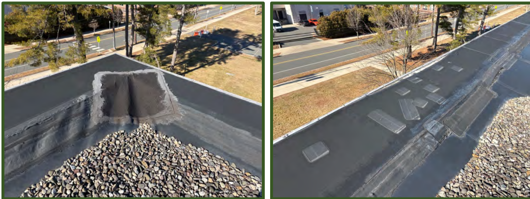
Figure 57-58 Seabrook Hall depicted, with patches and loose gravel which signify poor roof conditions 24
