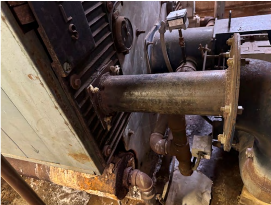
Boiler #2 FGR Piping - Improper Installation
