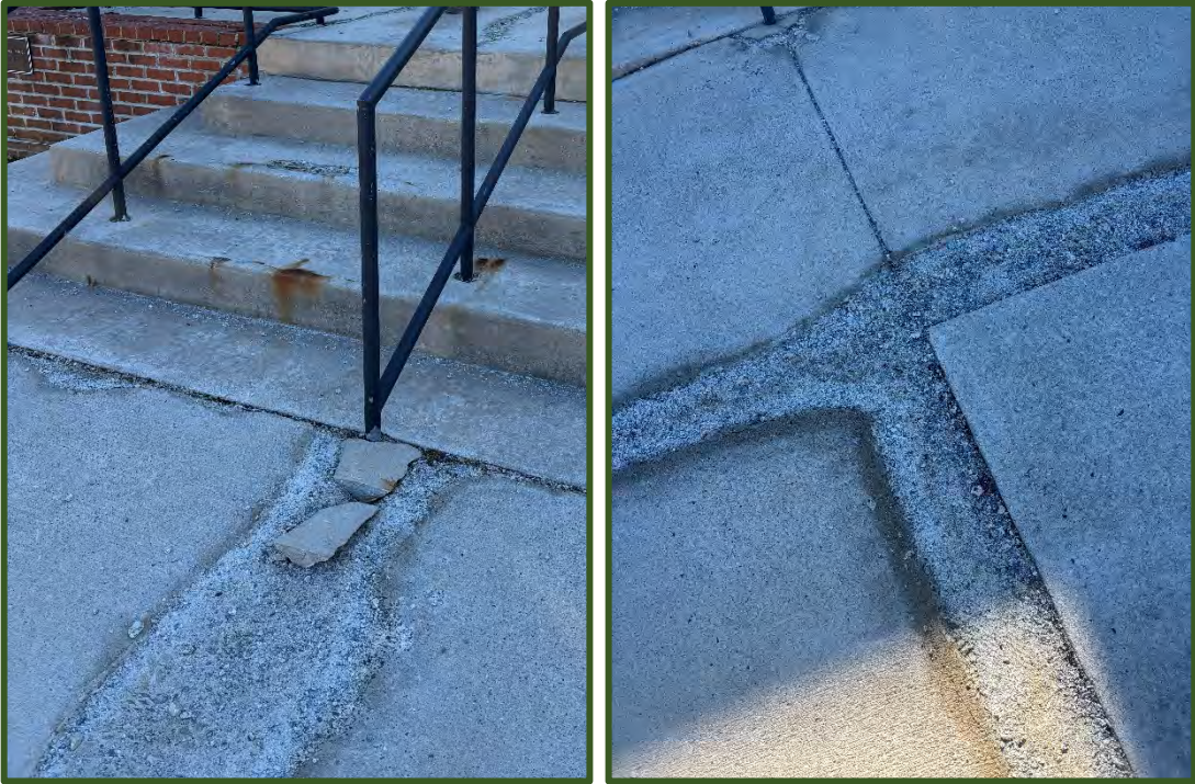
Figure 65-66: Cracked sidewalk outside of Hillman Hall and the Playhouse.
