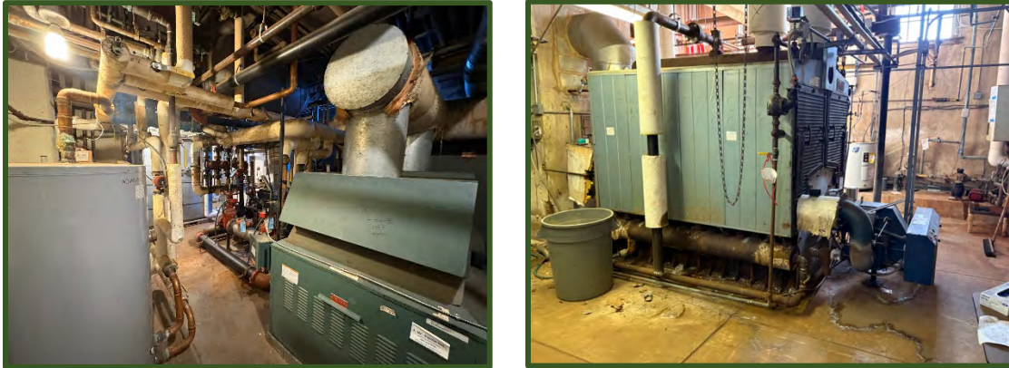
Figure 55 (left and right, above): System which services Dayton, Princeton and Ithaca Halls.
