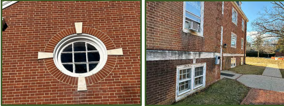
Figure 62 (left): Exterior rotted window at Bristol Hall. Figure 63 (right): Exterior rotted windows in Erdman Hall.
