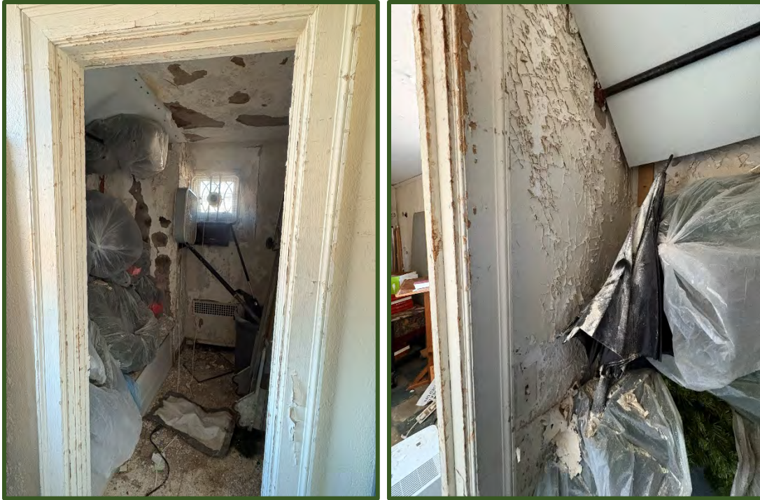
Figure 41-42: Steam damage depicted in Bristol Hall.
