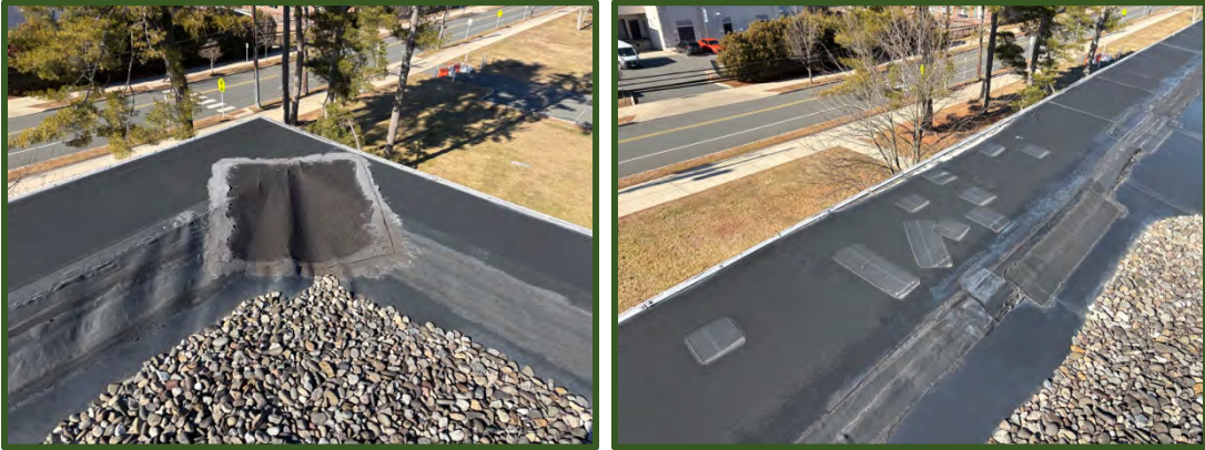
Figure 57-58 Seabrook Hall depicted, with patches and loose gravel which signify poor roof conditions 24
