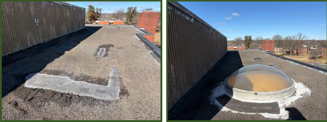
Figures 59-60: Roof of Student Center, depicted patches which signify poor roof conditions
