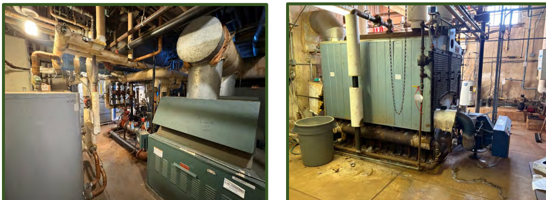
Figure 55 (left and right, above): System which services Dayton, Princeton and Ithaca Halls.
