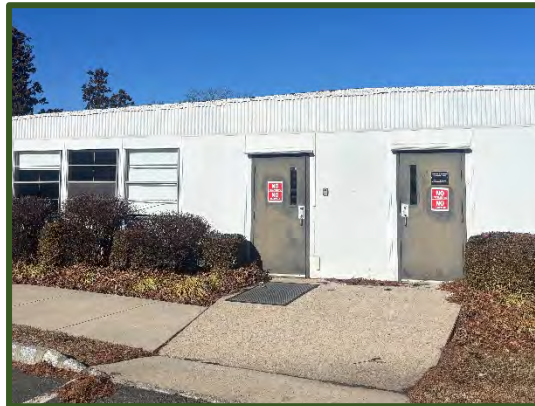
Figure 61: Relocatable Classrooms depicted, currently with a temporary roof that needs to be replaced.
