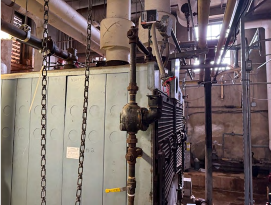
Boiler #2 LWCO Head - Replacement Required
