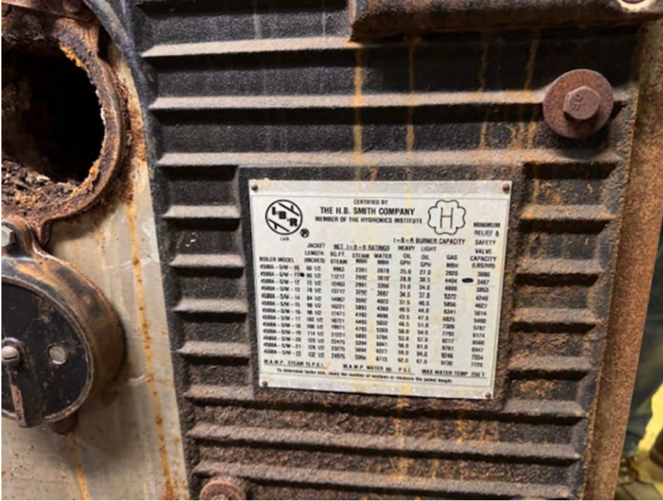
Boiler #1 Section Failure - Unit Offline
