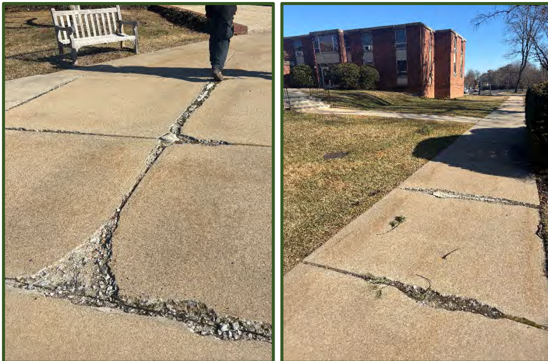
Figure 67 (left): Cracked sidewalk outside of Talbott Library. Figure 68 (right): Cracked sidewalk outside of dorm buildings.
