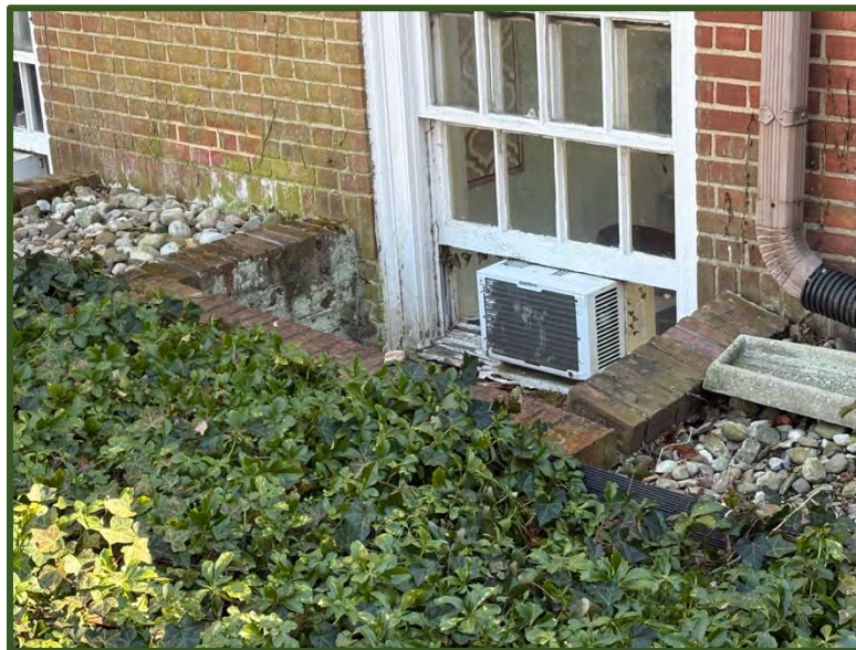
Figure 64: A window well in Williamson Hall depicted in dilapidated condition
