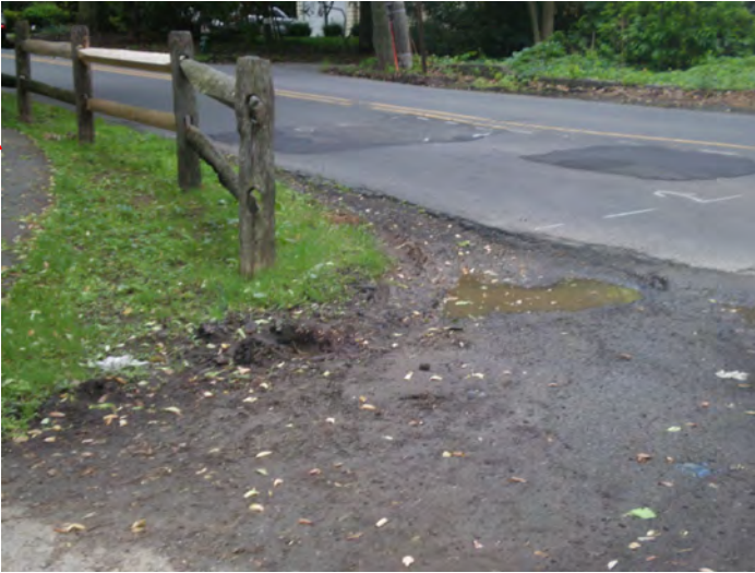
Paved entrance to the Park is in disrepair and needs to be attended to
